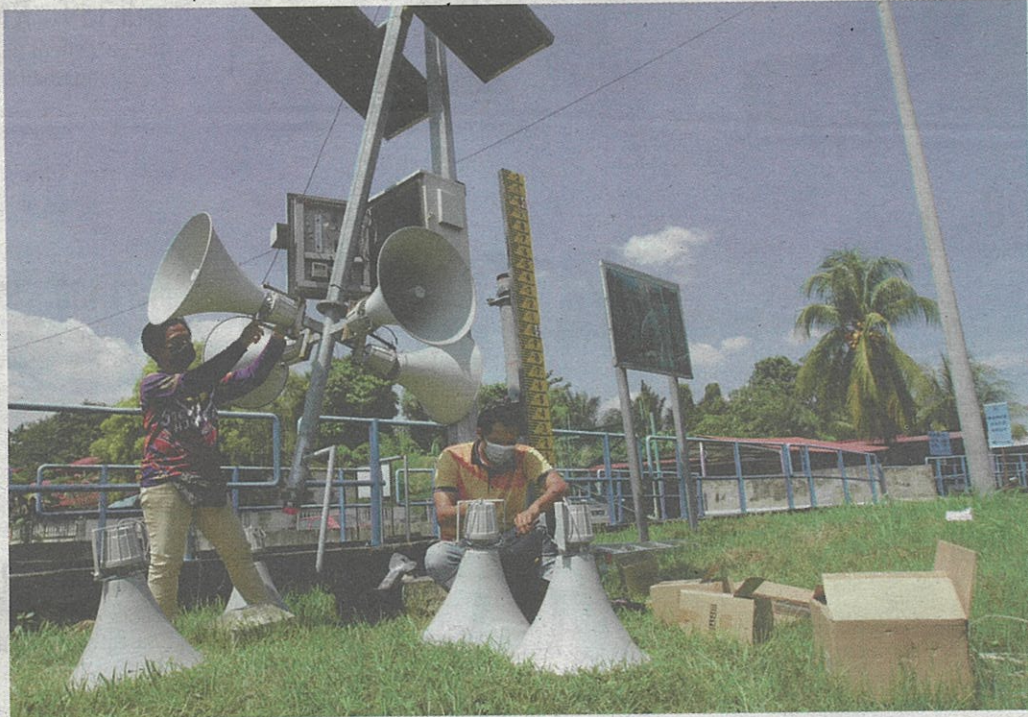
Repair works: DID contractor workers repairing and changing the warning sirens of the Flood Siren Warning System in Taman Maznah, Klang.
